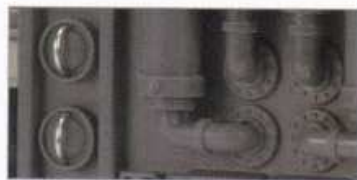
These lights have additional protection, made from fuse wire rods.
